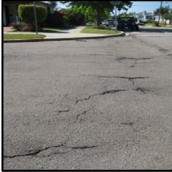
Poor crossing surface
